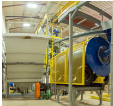
Image of Custom Clarifier installed 10 weeks after design authorization.
