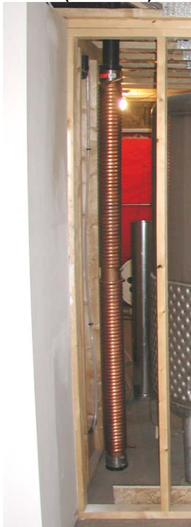
Figure 1a. Drain water heat exchanger in the Factor 9 Home Basement
