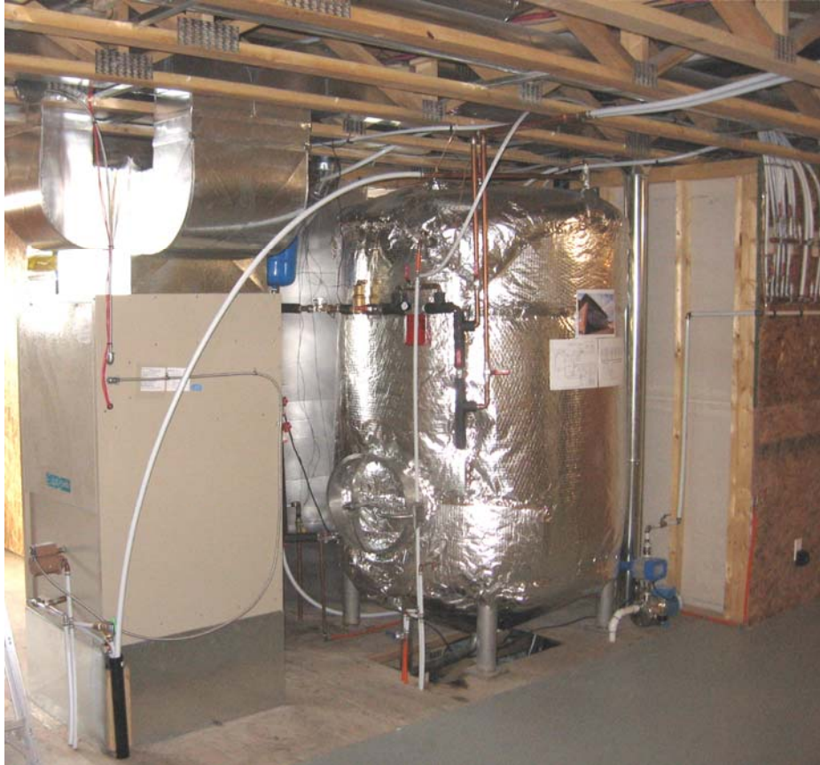
Figure 7. Fan coil with water to air heat exchanger and brushless DC fan motor on the left. Hot water is taken from the insulated storage tank and run through the fan coil to provide space heating for the house. In addition, the fan coil in the cooling season will take cool water from the pilings beneath the house to provide space cooling.
