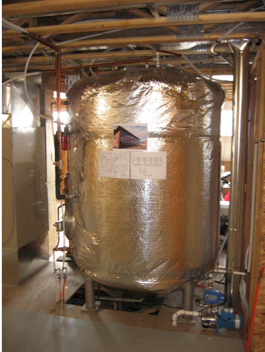
Figure 6. Insulated recycled stainless steel water storage tank (2350 Litre) to store heated water from the active solar heating panels.
