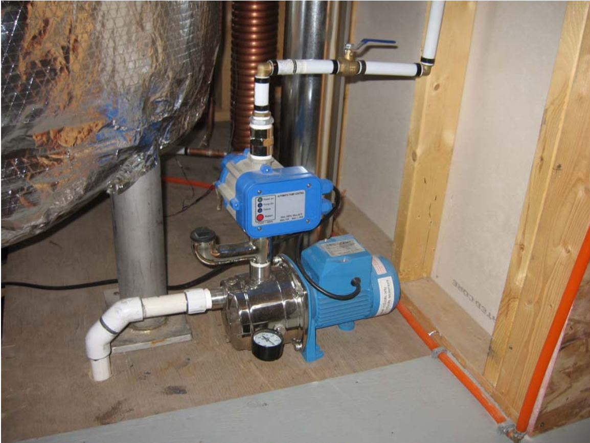
Figure 10. Pump that moves water from the 19,000 litre membrane tanks beneath the crawl space to the toilets and the exterior water uses.
