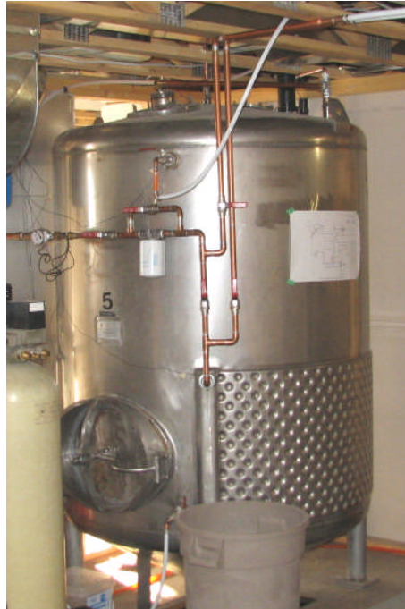
Figure 3. Heat storage tank for the solar heating system. The tank has a volume of 517 imperial gallons ( 2347 litres) Note the wrap around heat exchanger on the lower right half of the stainless steel tank. The glycol solution from the solar panels transfers heat to the tank via this heat exchanger. In an earlier life this tank was used in a brewery.
