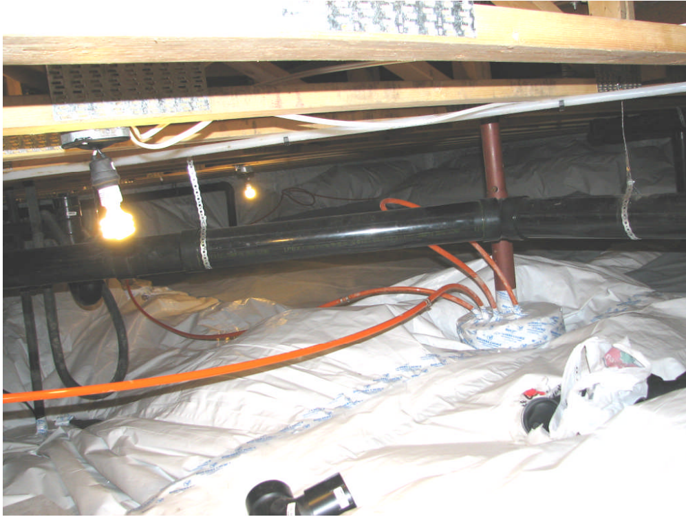
Figure 5. View of the crawl space beneath the basement floor. A very high degree of air sealing was accomplished with the ground cover membrane. This excellent air sealing will be valuable in limiting radon gas entry into the living space. The orange pipes are the plastic pipes that will extract cooling from the concrete pilings that support the house.
