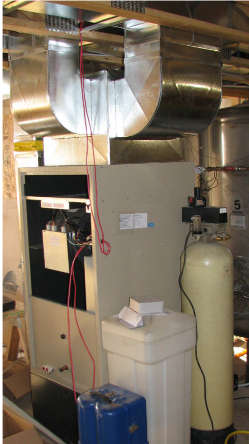
Figure 7. Air handler for the house. The unit has a brushless DC fan motor. An A coil ( water to air heat exchanger) is located in the lower part of the unit. The unit provides space heating by taking hot water from the large storage tank. In the cooling season, it will take cool water from the piping embedded in the concrete piles and the grade beam.
